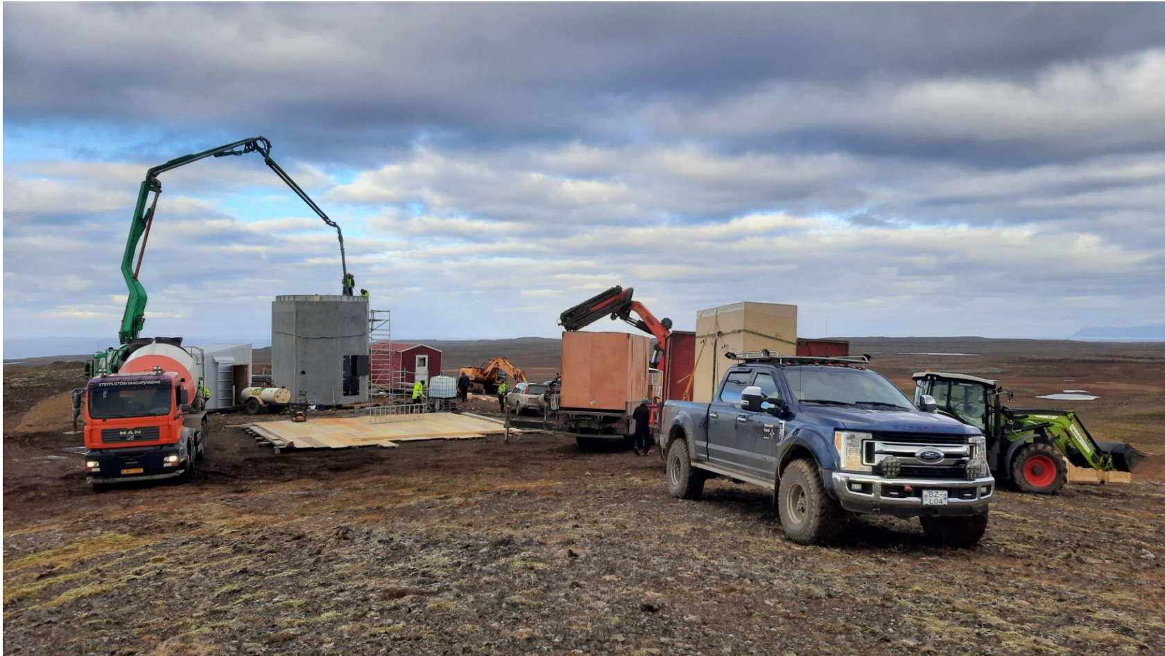
Construction of the radar tower at Skagi (66°N, 20°W, 160 m asl.). Photo Baldur Bergsson 21 Sept. 2022.
